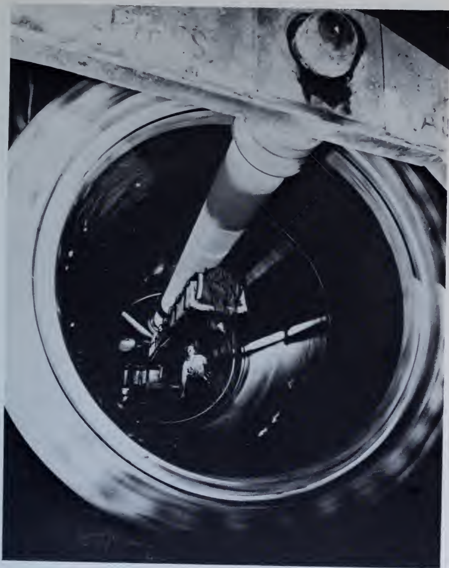
Figure 166. —Uniform placing of concrete in a rotating pipe form by use of a traveling belt conveyor visible at left center of form P830-D-17023.
